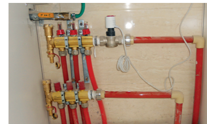
Danfoss manifold with RA-G valve and TWA-A actuator. This combination was installed in the smaller apartments to provide central temperature control via a CWD thermostat in the main living room. Individual room controls were installed in the larger apartments.
