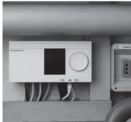
District Heating Controls
