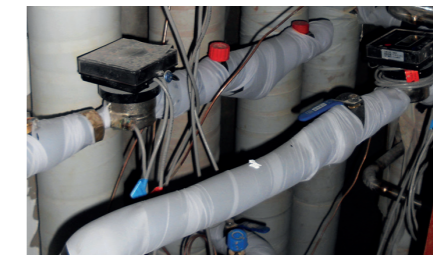
Danfoss ASV balancing valves and energy meters were installed in the technical room for each group of four apartments.
